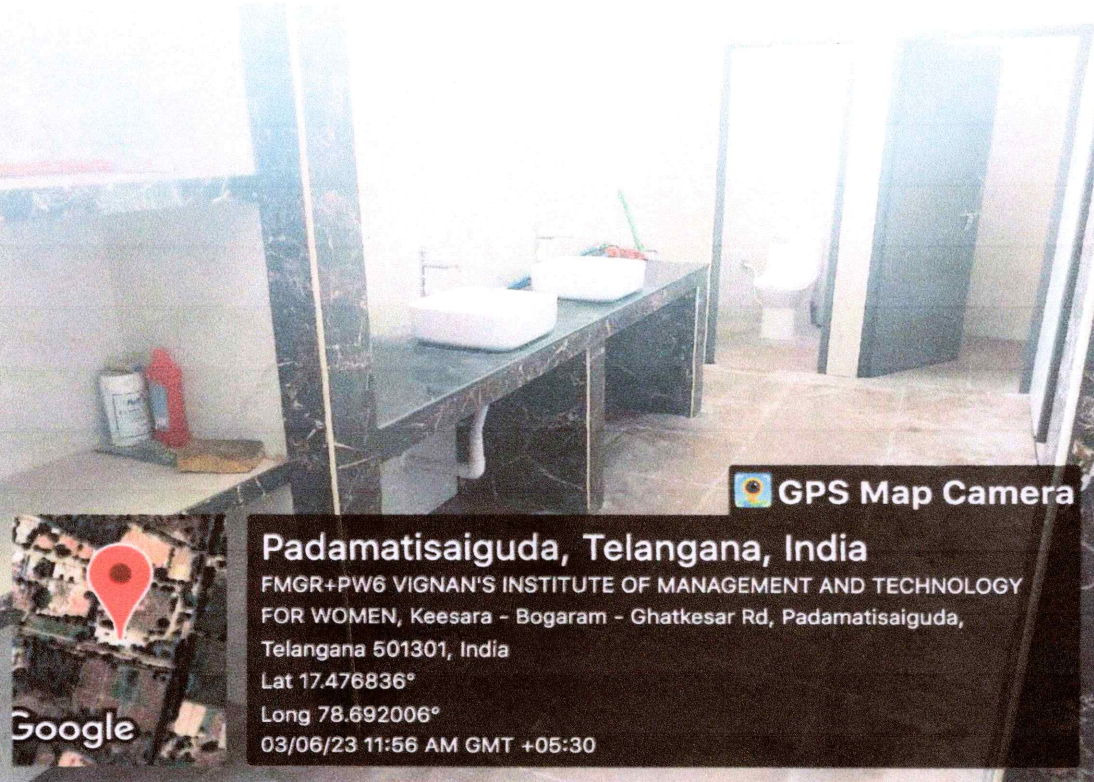
Disable friendly wash room
